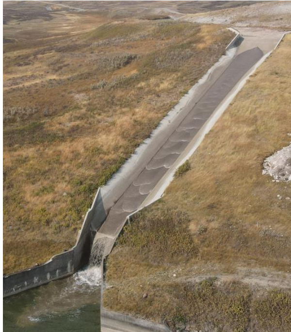
Figure 2-13. Drop 4 Chute Condition 4
