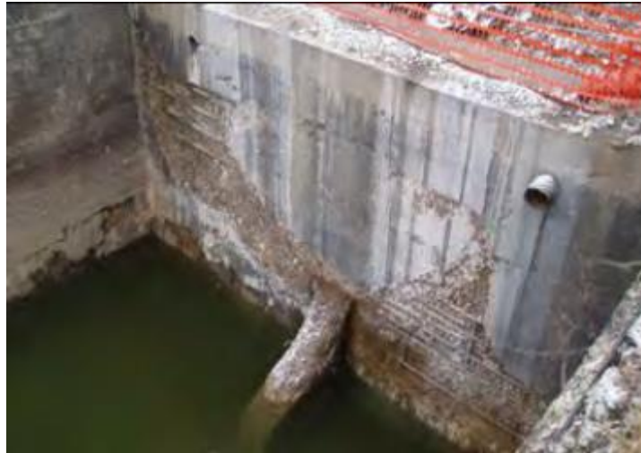
Figure 2-12. Drop 3 Plunge Pool Headwall Condition
