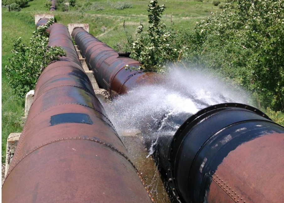
Figure 2-4. St. Mary Siphon Leaking Steel Barrels
