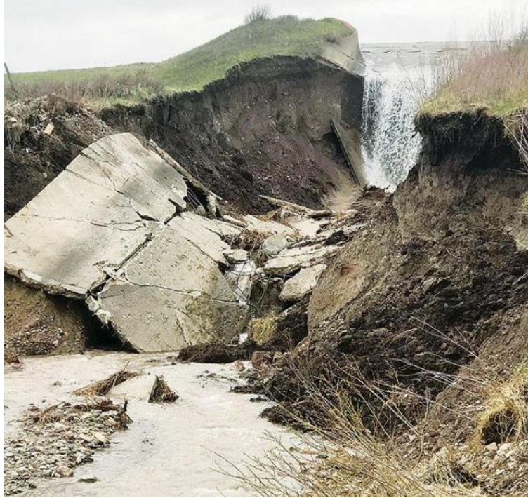
Figure 2-10. Drop 5 Failure on May 17, 2020 3
