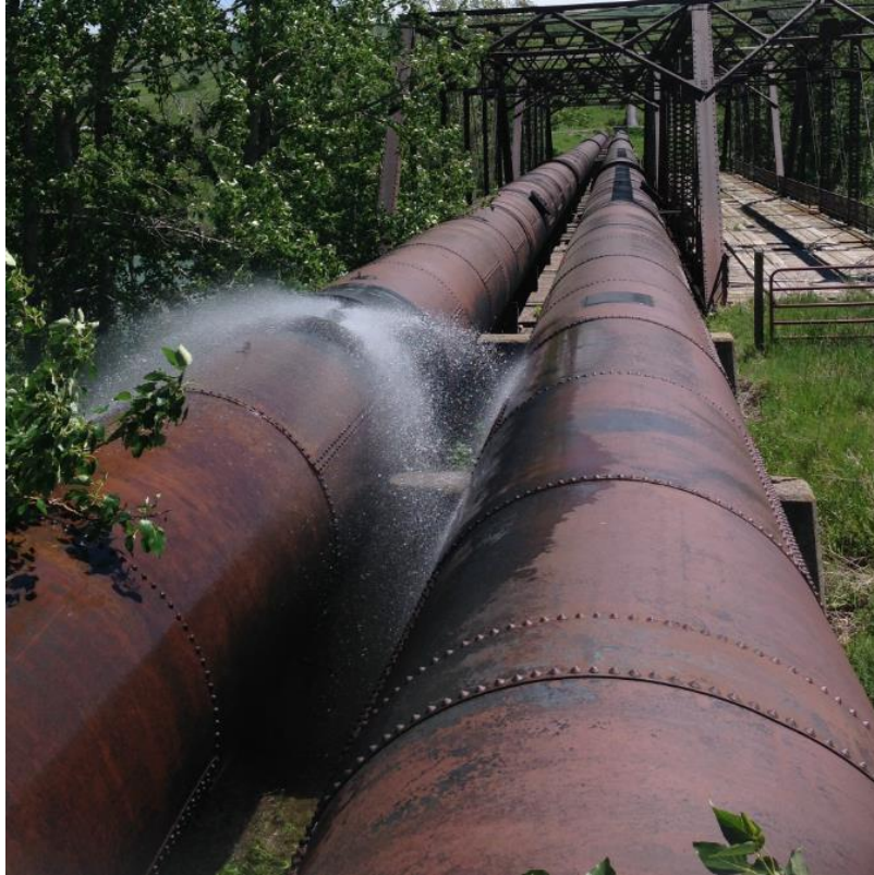
Figure 2-3. St. Mary Siphon Leaking Steel Barrels
