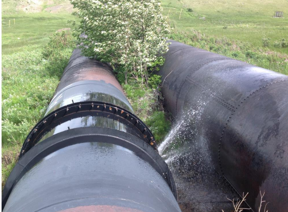
Figure 2-5. Halls Coulee Barrel Leak
