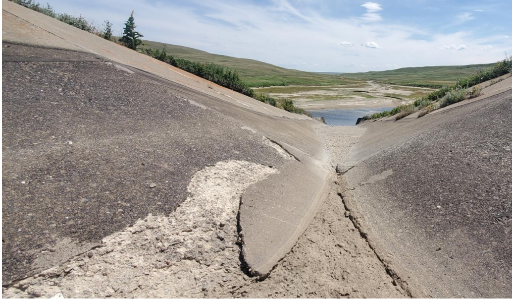
Figure 2-11. Drop 1 Chute Condition
