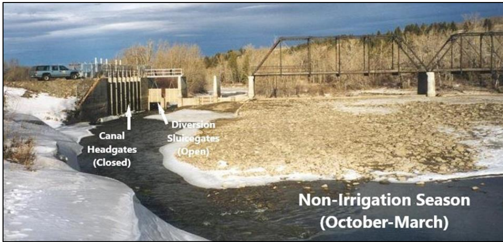
Figure 3. St. Mary Diversion Dam during the non-irrigation season. Photo taken from St. Mary River upstream of diversion dam and headworks (BOR 2020).
