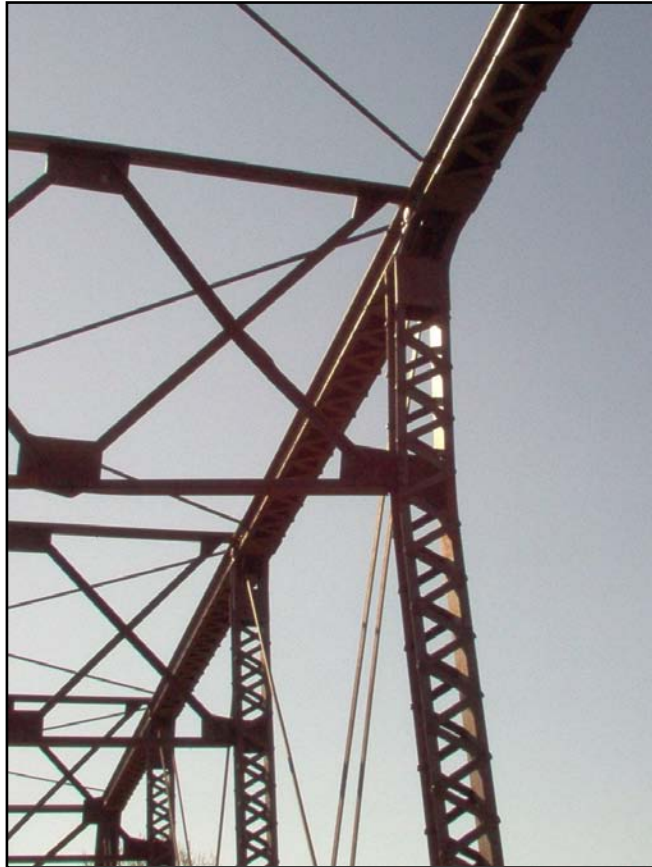
Photo 29. Damage to vertical truss (5/10/07).
