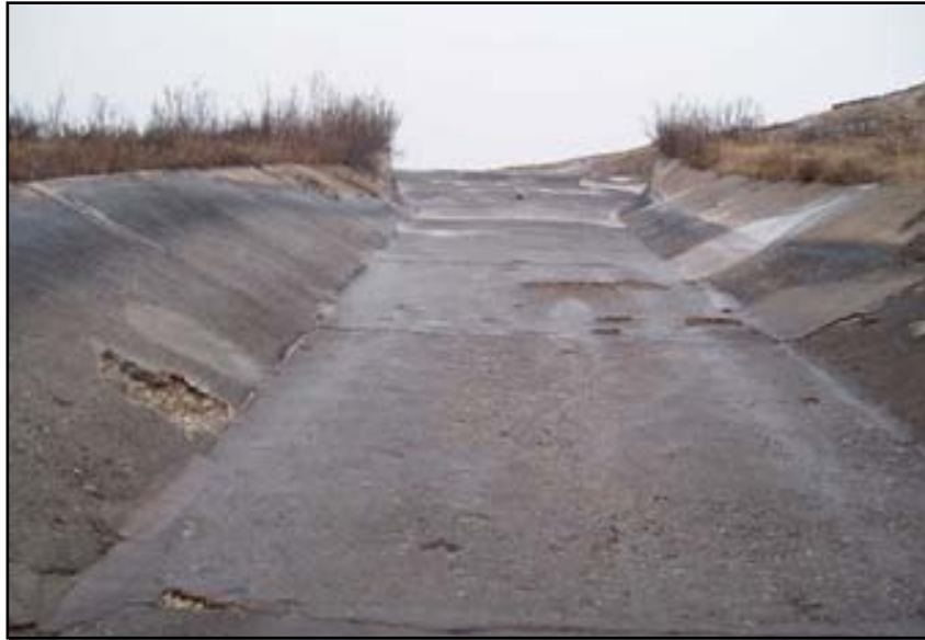
Photo 43. Close-up of concrete deterioration of Drop No. 4 chute floor (11/10/04).
