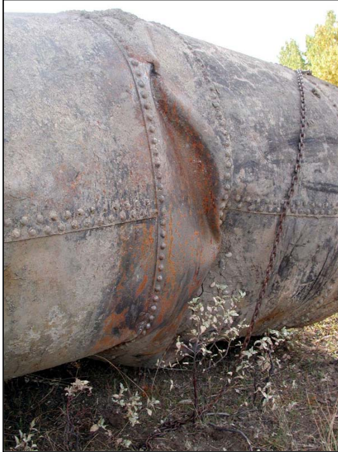
Photo 23. Photo shows buckled section of right pipe from the south slope that failed in 1996
