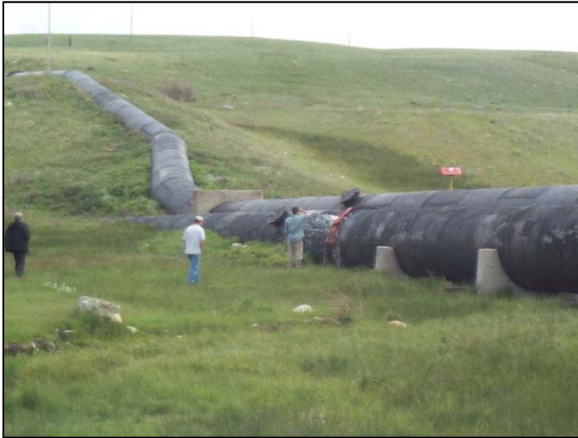
Photo 32. Looking downstream along the Hall Coulee Siphon at leaking expansion/contraction joint (06/24/04),
