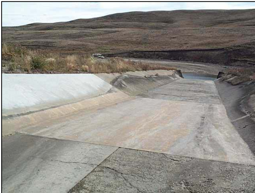
Photo 37. Drop No. 2 in the off-season. Note clean flow lines over new concrete surfaces replaced in 2002 and increased flow depth over rougher, older concrete surfaces (10/13/04).
