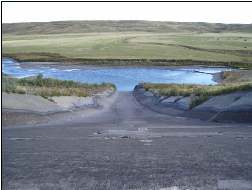
Photo 39. Downstream view of Drop No. 5. Note irregular flow regime and potential chute jumping as evident from the concrete staining (09/27/07).
