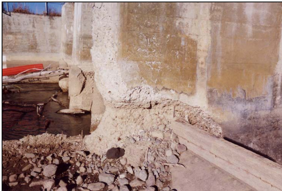
Photo 7. Looking west at upstream edge of sluiceway piers. Note concrete condition and exposed reinforcement (11/11/04).
