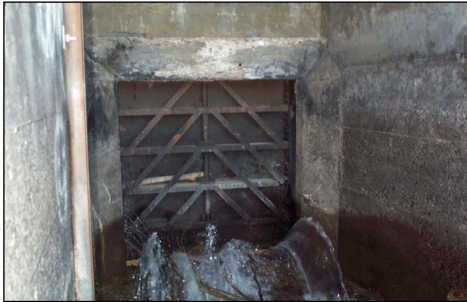
Photo 9. Close-up (downstream) of heavy leakage and debris at Gate 3 (10/13/04).
