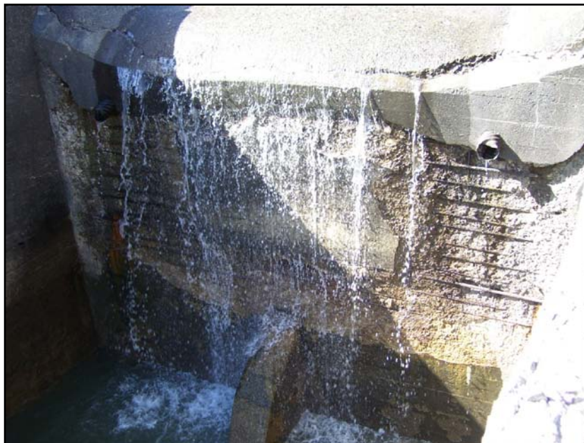
Photo 45. View of plunge pool headwall of Drop No. 1. Note condition of concrete and exposed reinforcement steel (09/27/07).
