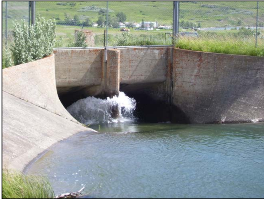
Photo 25. Close-up of St. Mary River Siphon inlet during diversion. Note stop log guides in concrete (07/18/08).
