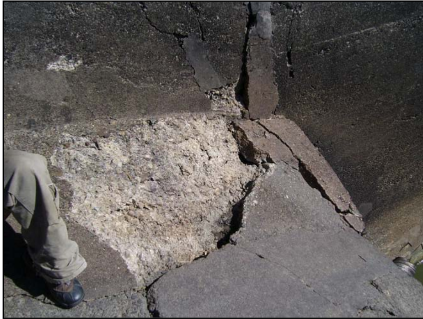
Photo 41. View of chute floor directly above plunge pool headwall of Drop No. 2. Note the degree of concrete ablation (09/27/07).
