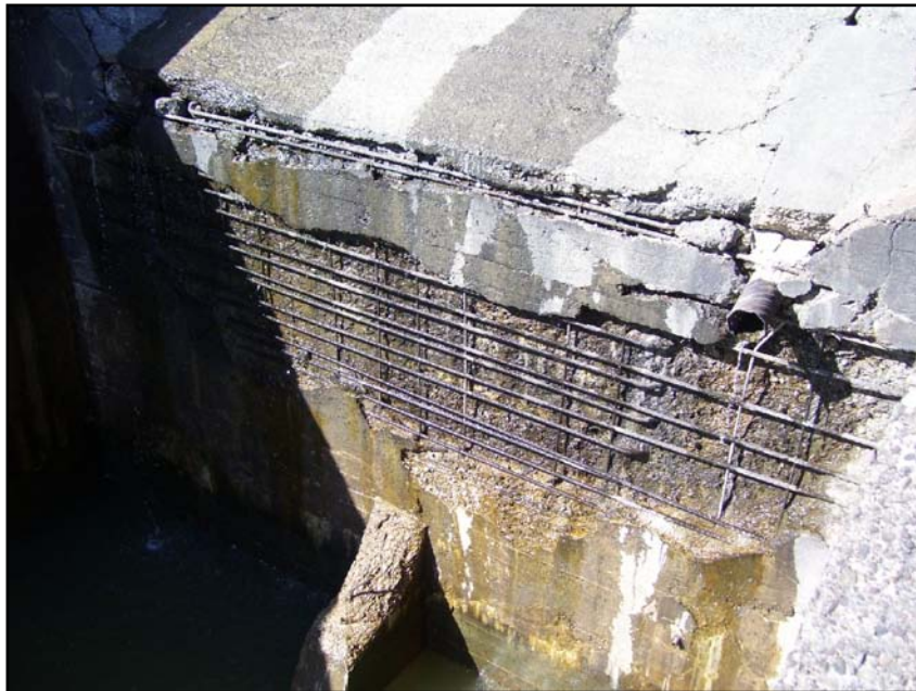
Photo 46. View of plunge pool headwall of Drop No. 2. Note condition of concrete and exposed rebar (09/27/07).
