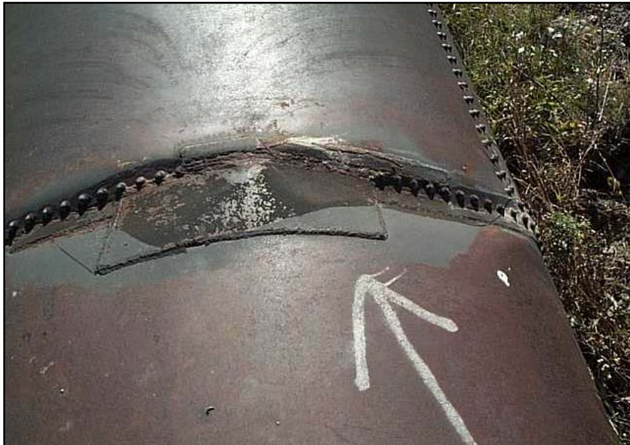
Photo 21. Typical siphon repair due to deflection and/or corrosion at a riveted joint. (10/13/04).
