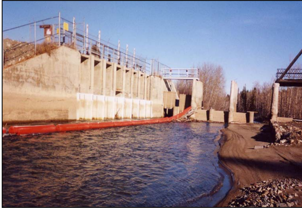
Photo 4. Upstream view of headgates showing trash boom, electric fish barrier, and dam sluiceways (11/11/04).
