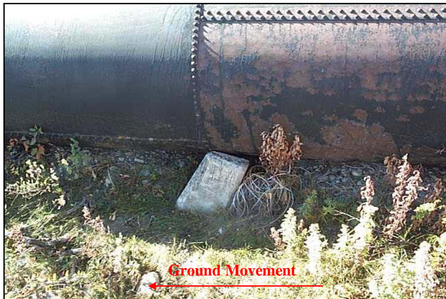
Photo 22. Photo shows ground movements right to left causing rotation of concrete support and point-loading of siphon which can lead to localized buckling (10/13/04). Photo shows the left side of the right barrel on the north slope of the St. Mary River crossing. The arrow points downhill.
