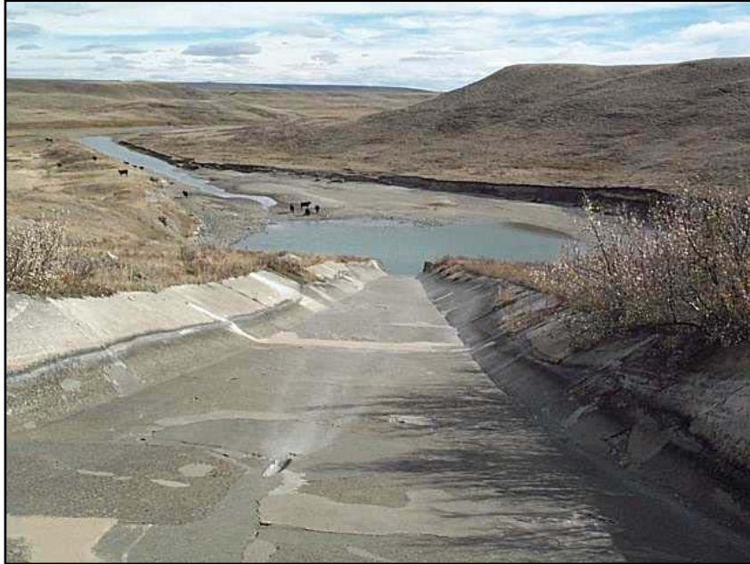
Photo 38. Downstream view of Drop No. 4. Note irregular flow regime and potential chute jumping as evident from the concrete staining (10/13/04).
