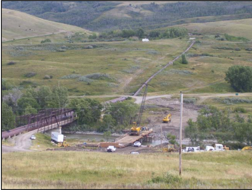
Photo 27. New Glacier County bridge under construction approximately 200 feet upstream of the existing St. Mary River Bridge (7/17/08).
