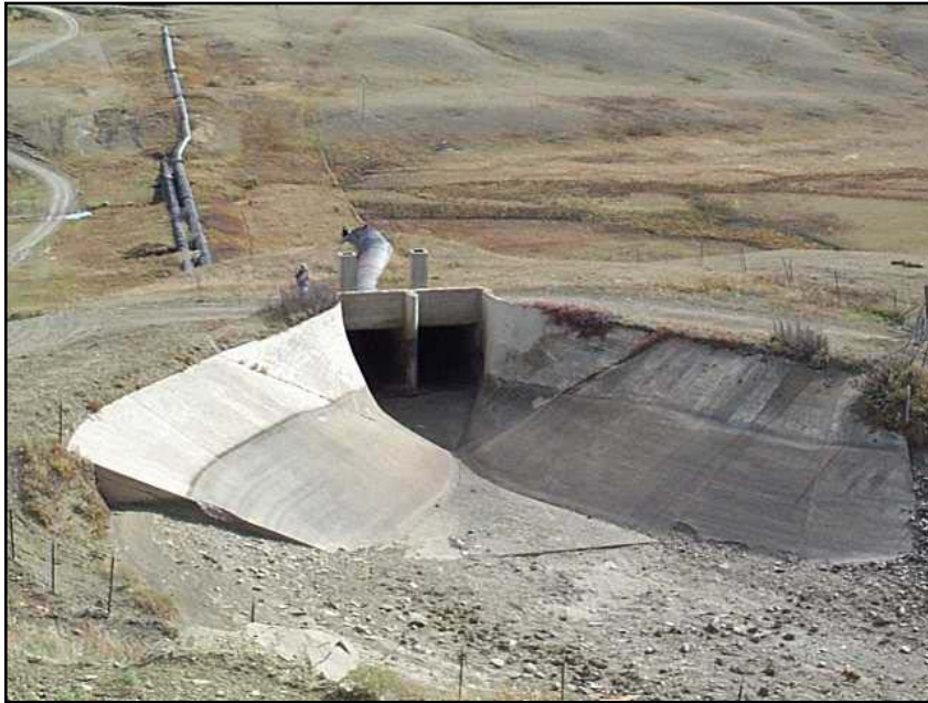
Photo 30. Looking downstream at concrete inlet transition structure for the Hall Coulee Siphon crossing (10/13/04).
