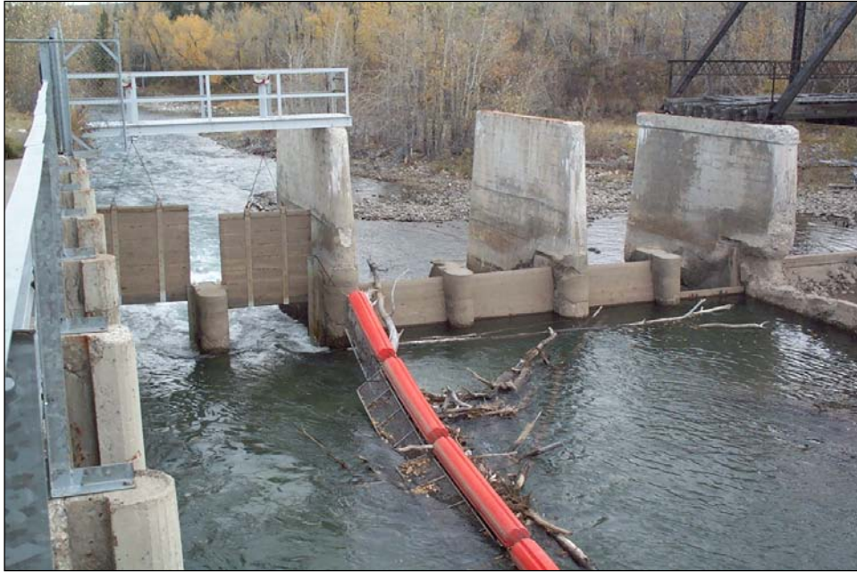
Photo 2. Looking downstream (north) at three sluiceways and 6 bays on the west side of diversion dam. Canal headgates are left of photo. Note two manually operated lift gates used to regulate flow and permit passage of off-season flow (10/06/04).
