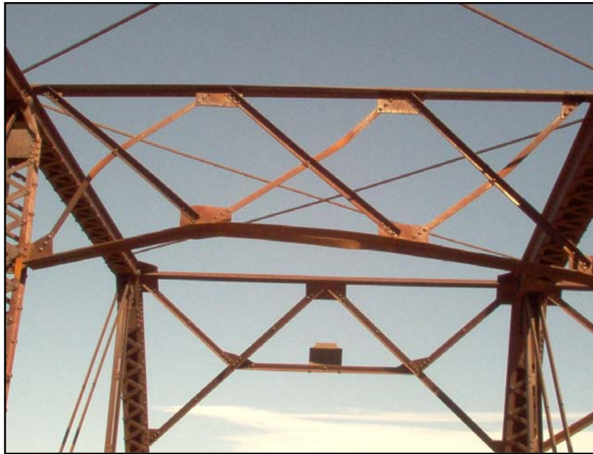
Photo 28. Damage to top chord (5/10/07).
