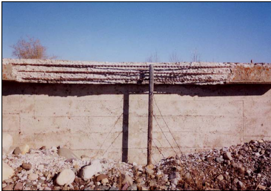
Photo 12. Kennedy Creek side of outlet transition structure. Note exposed steel reinforcement (11/11/04).
