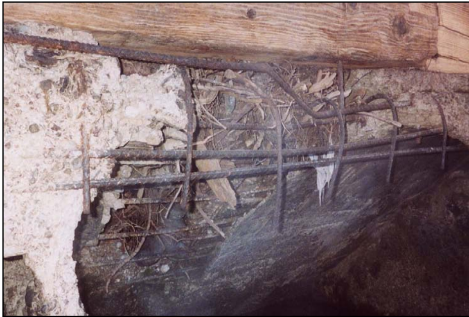
Photo 6. View of concrete condition of the underside of fixed weir portion of diversion dam (11/11/04).
