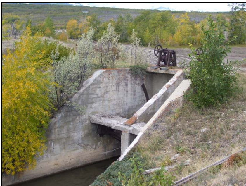
Photo 15. Downstream view of Kennedy Creek wasteway structure. Note condition of concrete surfaces (09/25/07).
