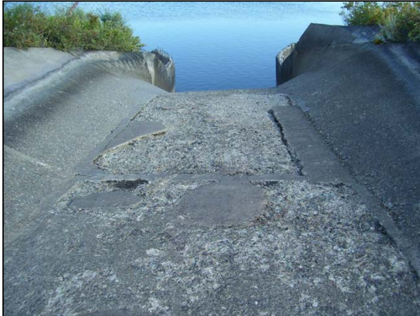
Photo 44. Looking downstream at lower end of chute floor for Drop No. 5. Note condition and surface roughness of concrete (09/27/07).
