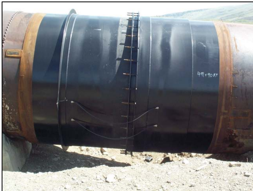
Photo 24. A typical expansion/contraction joint installed by USBR staff on the right pipe (5/16/06).
