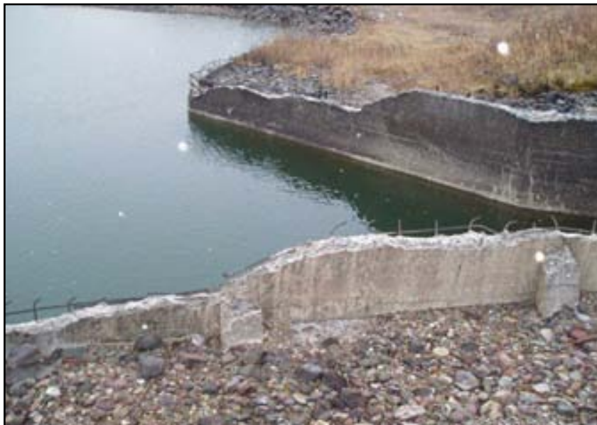
Photo 47. Heavily damaged/eroded wing and training walls on Drop No. 5 (11/10/04).
