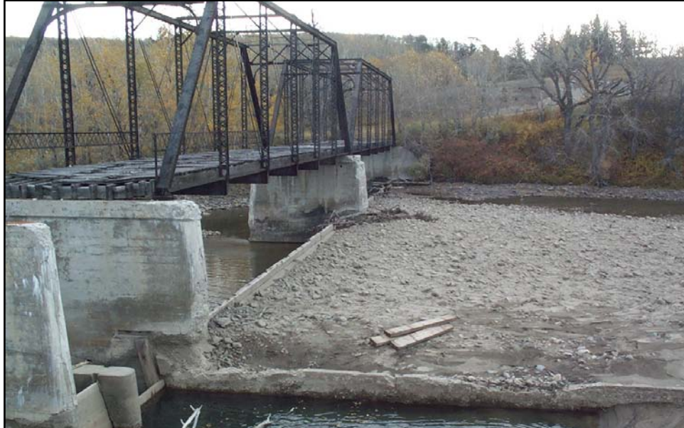
Photo 1. Looking east across St. Mary River during the off-season at the two fixed weir segments below the remaining bridge spans. Note condition of concrete, magnitude of sediment deposition upstream of dam and timber plank added to fixed weirs (10/06/04).
