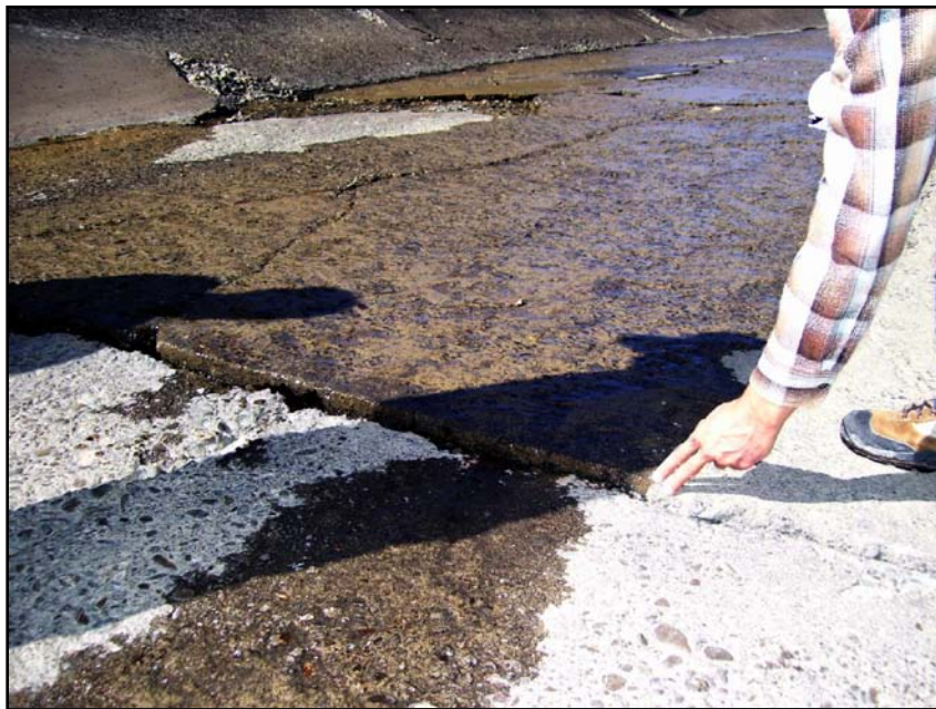
Photo 42. View of slab offset in chute floor of Drop No. 2. (09/27/07).
