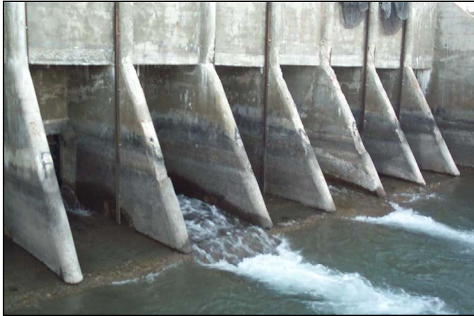
Photo 8. Downstream view of headgate structure during the off-season. Note heavy leakage through Gates 3 and 5 (10/13/04).
