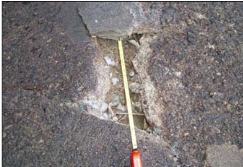
Photo 40. Close-up of concrete deterioration of Drop No. 4 chute floor (11/10/04).
