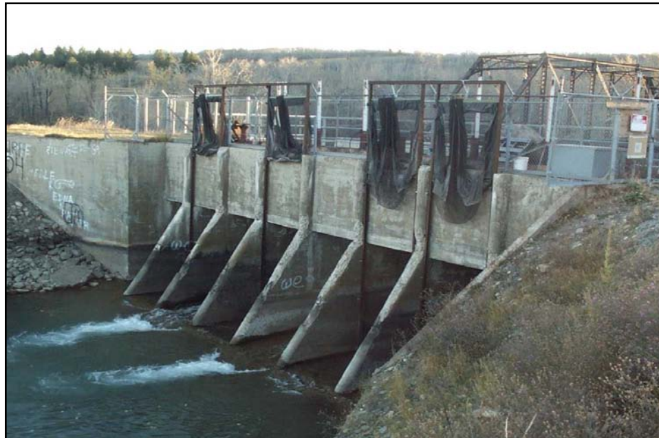
Photo 3. Looking at downstream end (canal side) of headgate structure. Diversion dam is located behind headgates (10/13/04).
