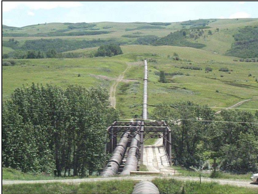
Photo 26. Looking downstream along the St. Mary River Siphon at the existing bridge (07/04/05).
